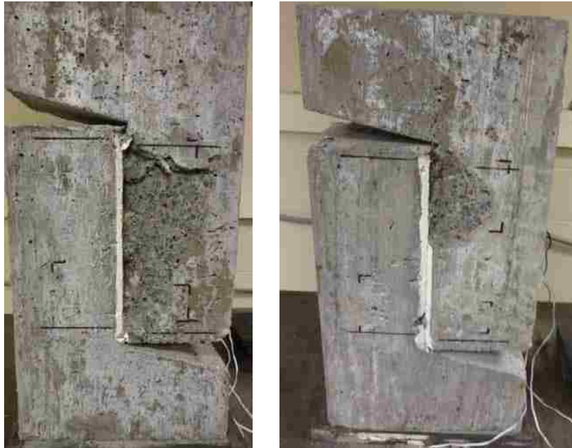
Figure 3.34 Concrete Cover Spalling Experienced by Specimen S-SL-CJ-S-1 (left), Specimen S-SL-CJ-S-2 (right)
