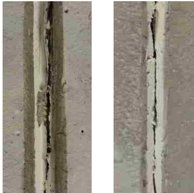
Figure 4.1 Typical Shear Plane Crack Normalweight Concrete Monolithic Interface (left), Shale Sand-lightweight Concrete Monolithic Interface (right)
